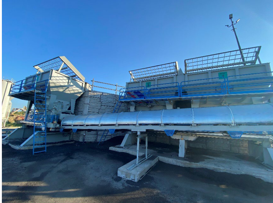
Figure 2 – RAP Cold Feed Bins at City Asphalt
